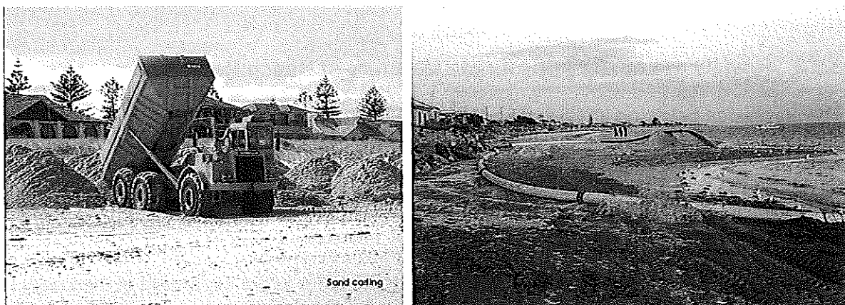
Figure 19 Examples of beach nourishment (left : Adelaide beach using sand carting and right – Lucky Bay using a dredge and pipeline).
